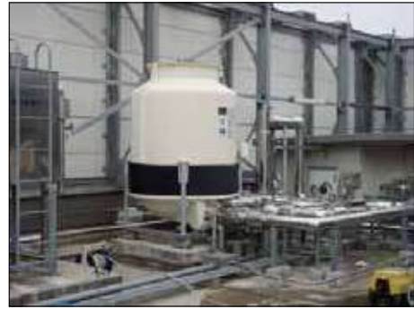
Cooling Tower C
