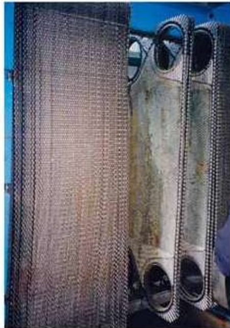
CONTROL OF HONEY COMB FILL OF COOLING TOWER
