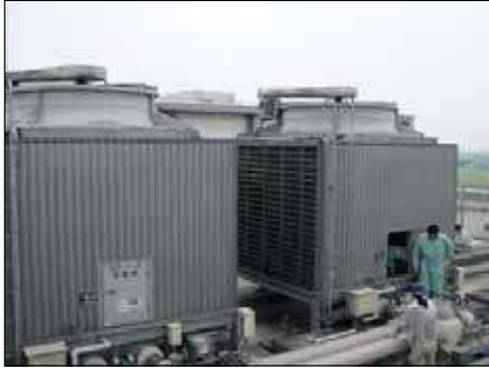
Cooling Tower A
